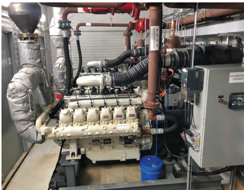
Interior of the power-generating unit located outside the arena.
